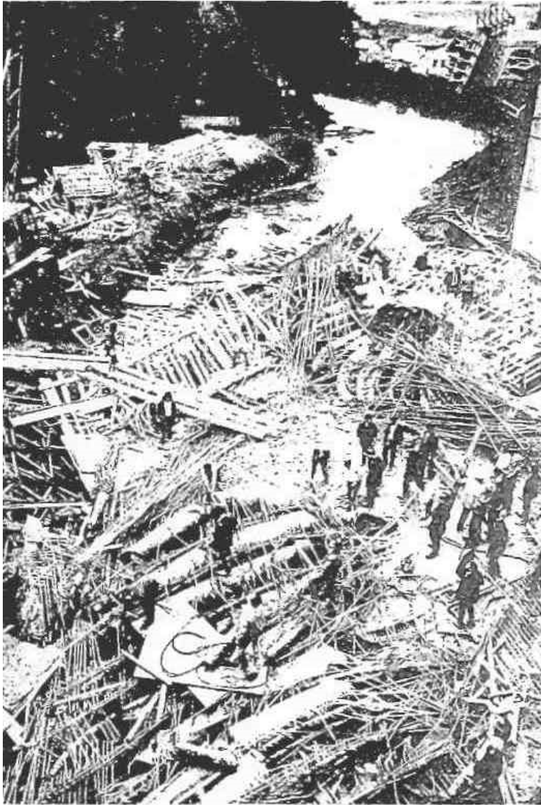
A GENERAL view of the tons of crumbled scaffolding which crashed forty feet into the River Lodden.
