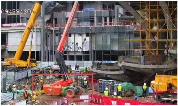
Missing warning lines
