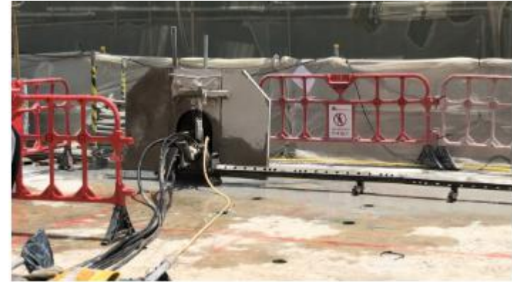
Using saw cutting machine to cut the existing slab to minimize air, noise and vibration impact
